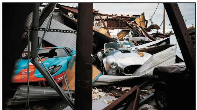
A metal frame building after hurricane Michael... not a good thing for your classic cars.
